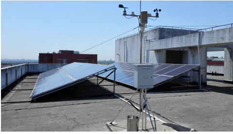
Fig. 9. PV array installed at ECUST, Shanghai.
